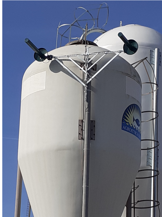
Figure 3: Gateways and their antennas in the installation site.
